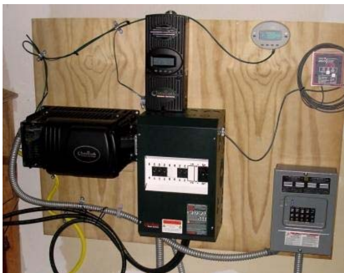
The control panel.
