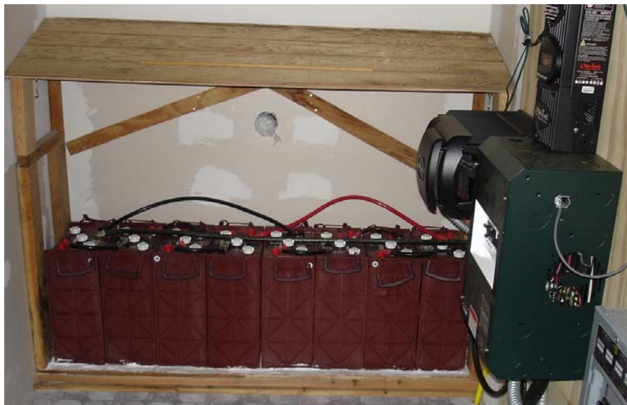
Eight Trojan L16HC batteries. The white powder at the base is baking soda, which is cheap insurance against a future spill. The battery-box fan is not yet installed.
